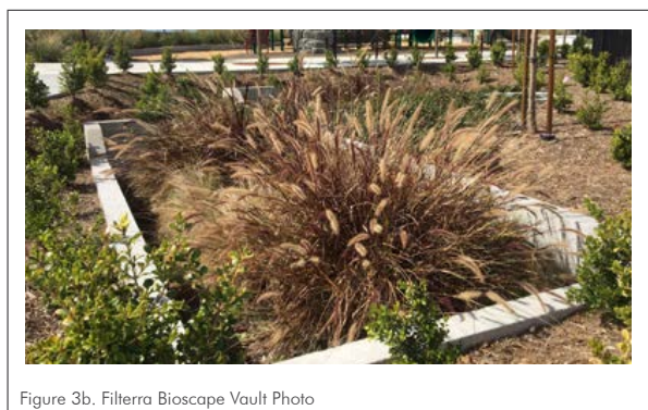
Figure 3b. Filterra Bioscape Vault Photo
